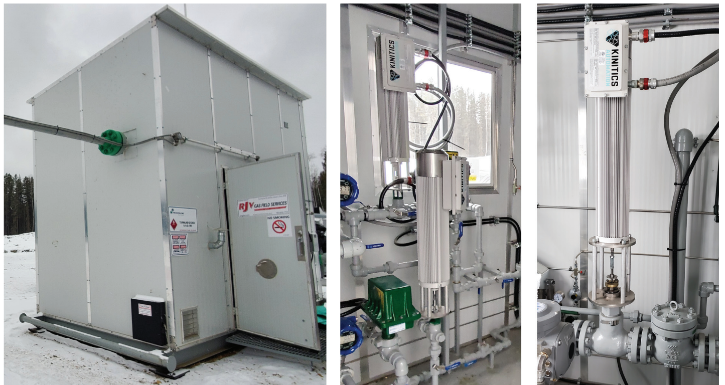
Figure 1: The KVA, an SMA bundled wire actuator, deployed at a natural gas production facility near Edson, Alberta.
